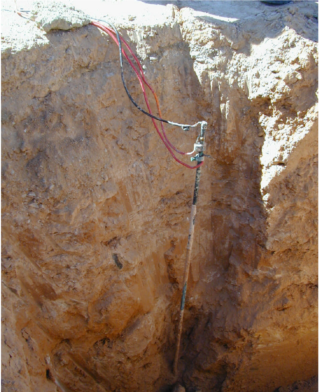
Figure 2. 5/8" x 8' copperbonded ground rod removed after 10 years (Pawnee Site).
